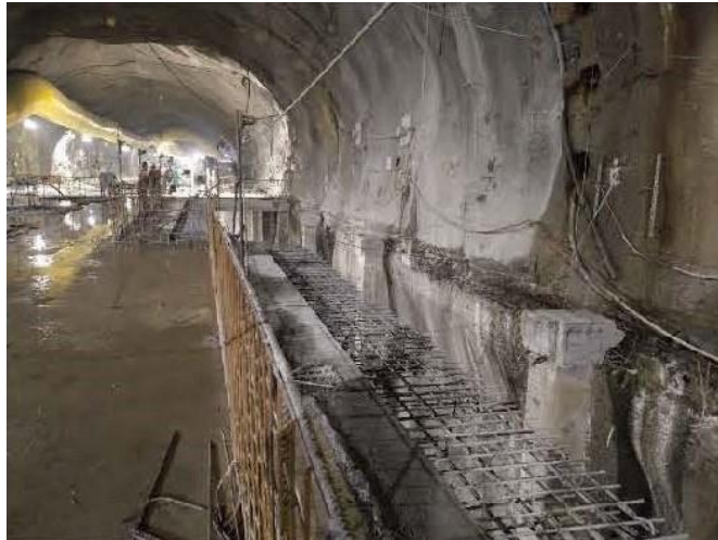
Figure 39: Ongoing civil works at the cable gallery before installation of cable trays and cables
