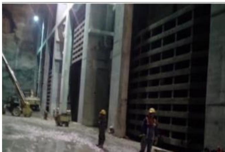
Figure 51: Draft tube gates (archive, picture taken before May 2018)
