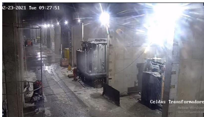
Figure 38: two single-phase transformers 3 and 4
