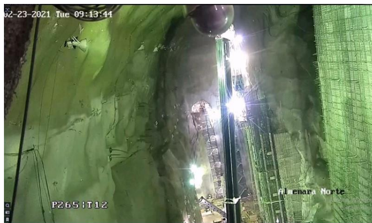
Figure 50: Ongoing installation of the guides of draft tube gates in the North Surge Shaft
