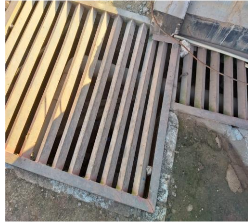
Oil and water separator at the Wash bay.
