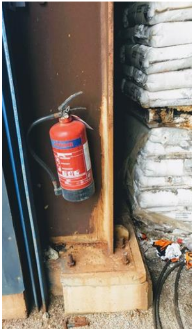
Fire extinguisher in the closed storage warehouse.
