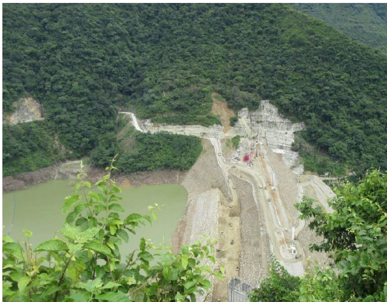
Figure 30 – Aerial view of left abutment. Geomorphology exposing no unstable forms. Skin slides only.
