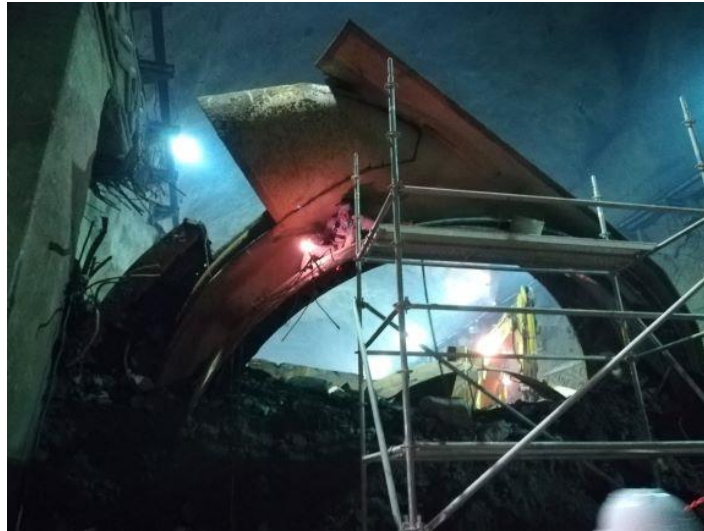
Figure 11 – Unit 2, stay ring displaced by water flood undercutting and removing.
