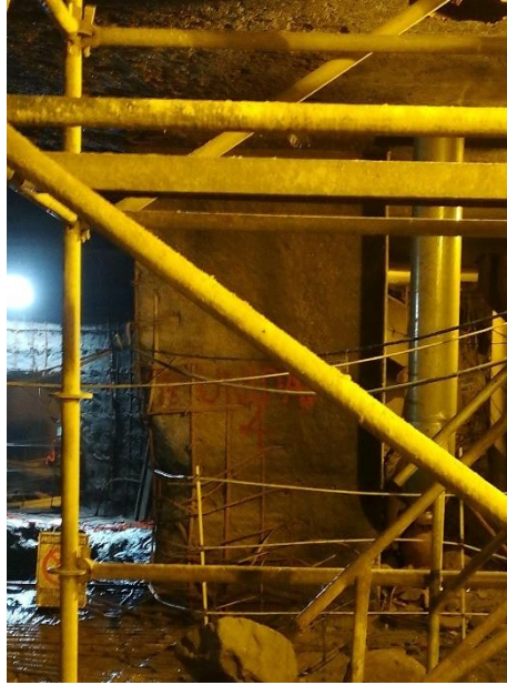
Figure 14 – Massive wall at draft tube cone level with exposed steel bars and signs of erosion in the lower left part.
