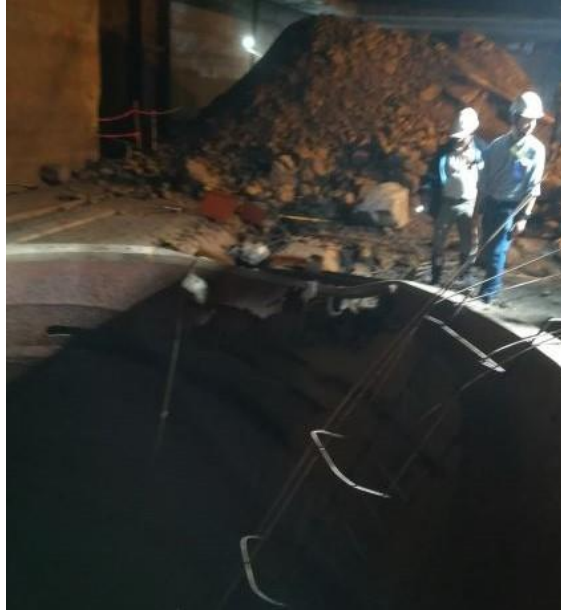
Figure 12 – Damaged Unit 3 draft tube.
