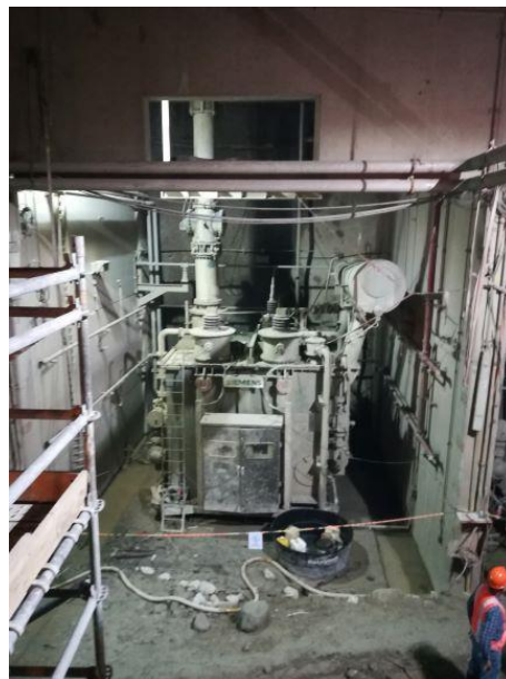
Figure 6 – One of the single-phase step-up transformers.
