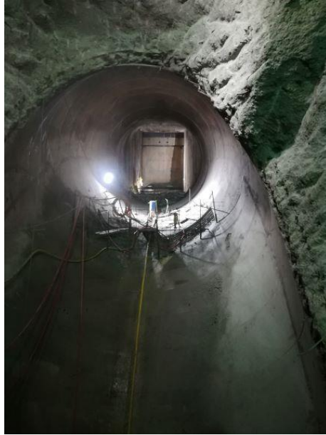
Figure 22 – Upper elbow of penstock n 1 “open” for facilitating installation of steel lining with on the background the downstream face of intake gate.
