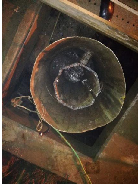
Figure 20 – Damaged and cut section of isolated phases bus duct of Unit 3.
