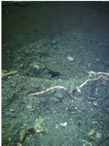
Figure 18 – The flange of turbine shaft emerging from the debris inside Unit 4 stator.
