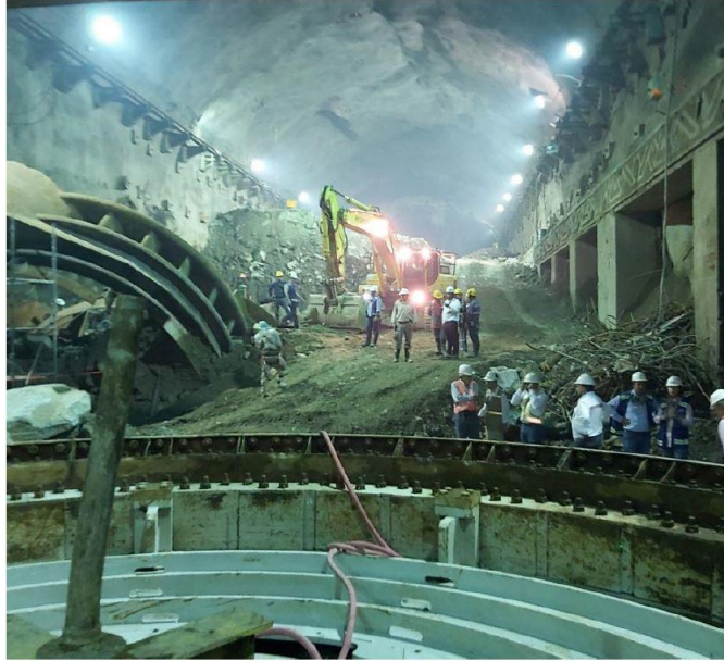
Figure 1 – PH cavern seen from the loading bar. Overall stability of the rock mass is recognized.
