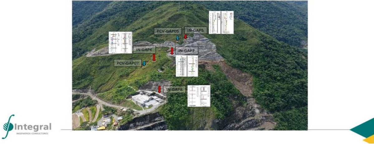
Figure 33 – Right abutment and zone over “El Romerito.” Position of inclinometers. Monitoring results are satisfactory. Only the IN-GAP-05, nevertheless over the terminal part of the natural slope, shows a displacement of about 1cm at a depth of 18m.
