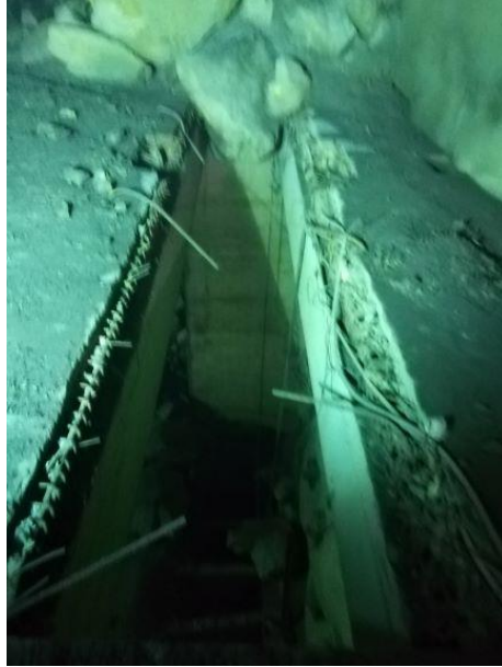
Figure 21 – Relatively well-preserved slot for Unit 5 draft tube gate in the south shaft chamber.
