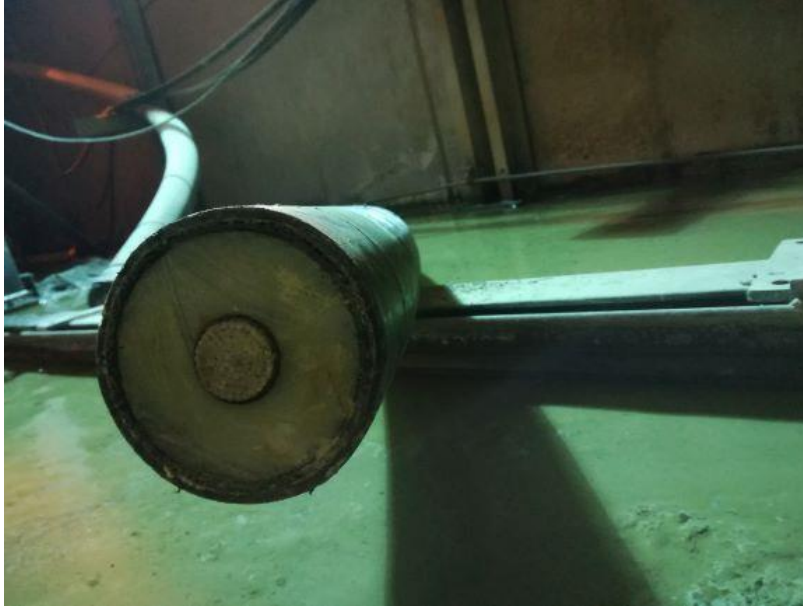
Figure 7 – One of the HV single phase cables.
