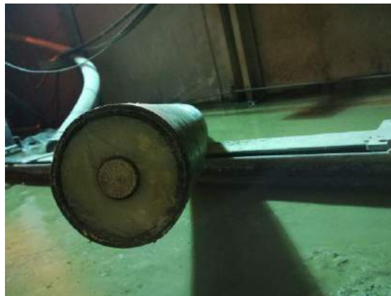
Figure 22: HV single phase cable[archive]
