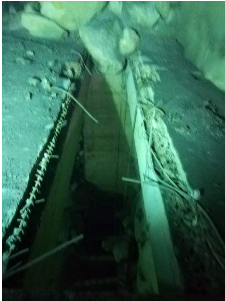
Figure 26: Slot for unit 5 draft tube gate in the south shaft chamber: guides are lost
