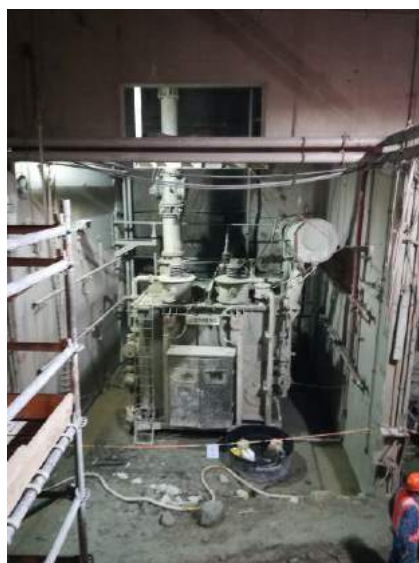
Figure 21: single phase transformer[archive]
