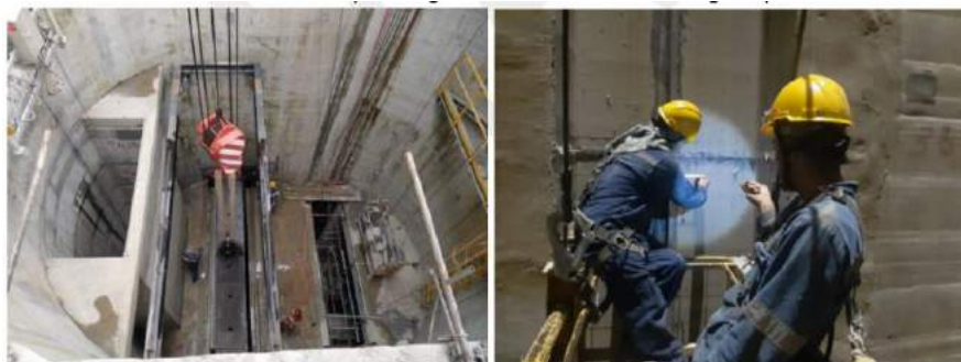
Fig. 28- Intake gates: Left, lowering gate 3 in its pit using temporary crane. Right: Inspecting guides of gates 5 and 6
