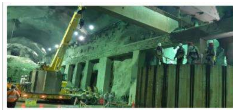
Figure 23: The second crane at work in the southern part of the powerhouse
