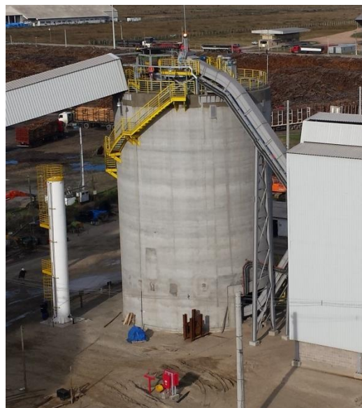
Figure 4 – Chips silos. Source: Pöyry, 2018.
