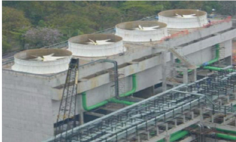
Figure 8 – Cooling tower. Source: Pöyry, 2018.
