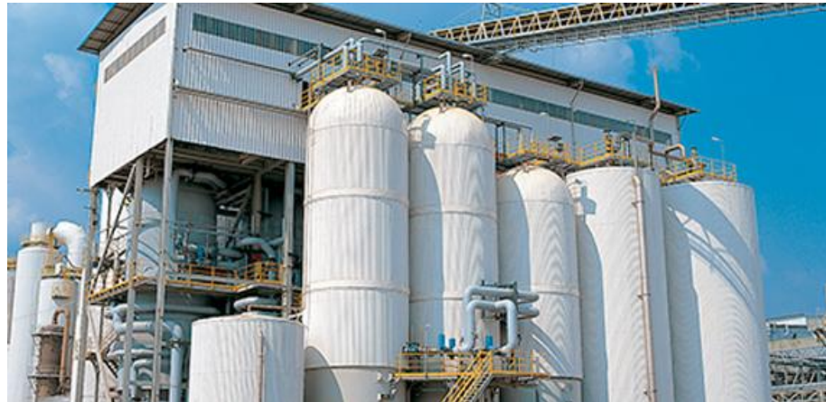
Figure 5 – Cooking Plant. Source: Pöyry, 2018.
