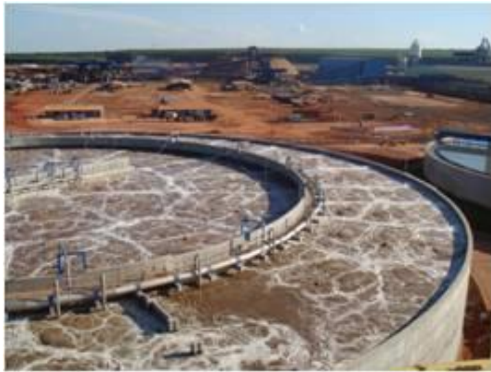
Figure 9 – Aeration tank. Source: Pöyry, 2018.
