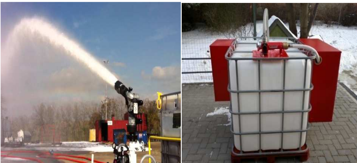
Photo 15 & 16 – Fire Hydrant with Monitor and Fire Suppression Foam Supply System
