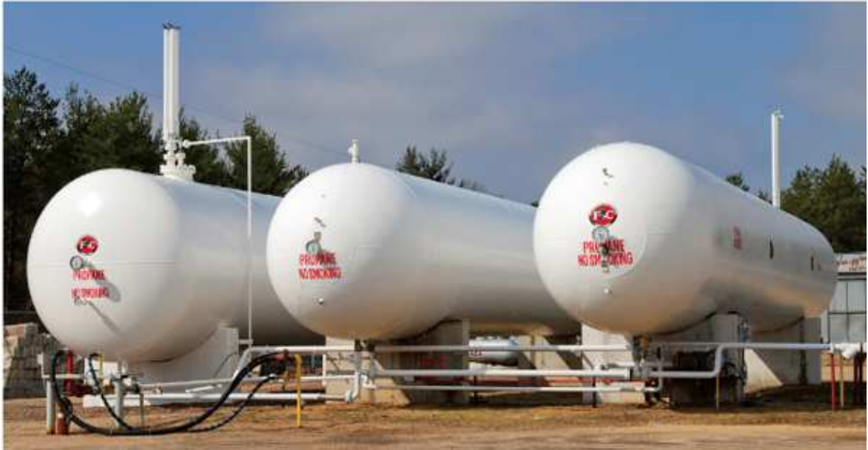
Photograph 11: LPG Tanks Interconnected with several pipelines
