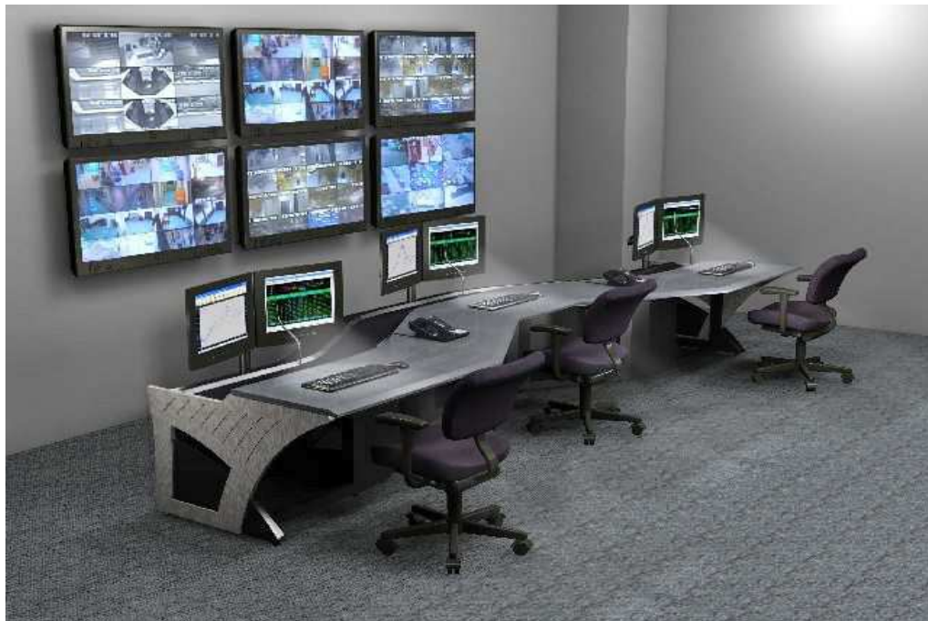
Figure 30: Example of a Control Room with Monitoring Displays
