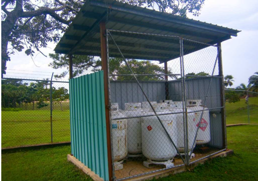
Photograph 39: Covered shed with adequate ventilation for the storage of Mercaptan Cylinders.
