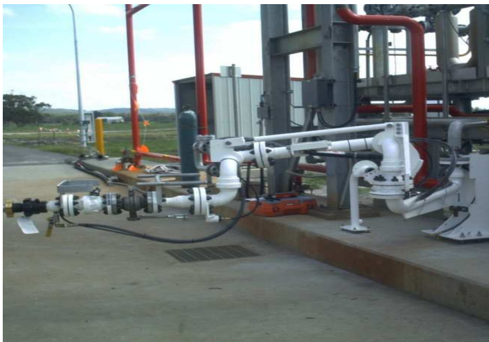
Photograph 20 A: Example of LPG Tanker Truck Loading Arm
