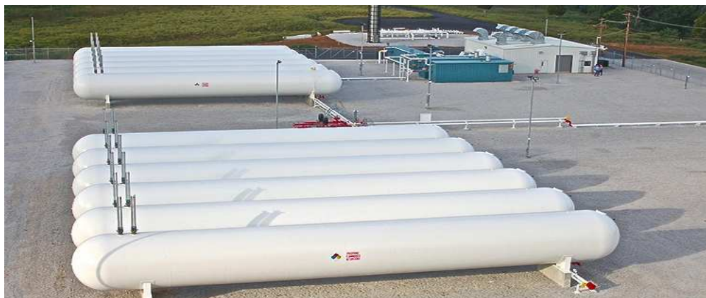
Photograph 3 – Example of 6-tank batteries
