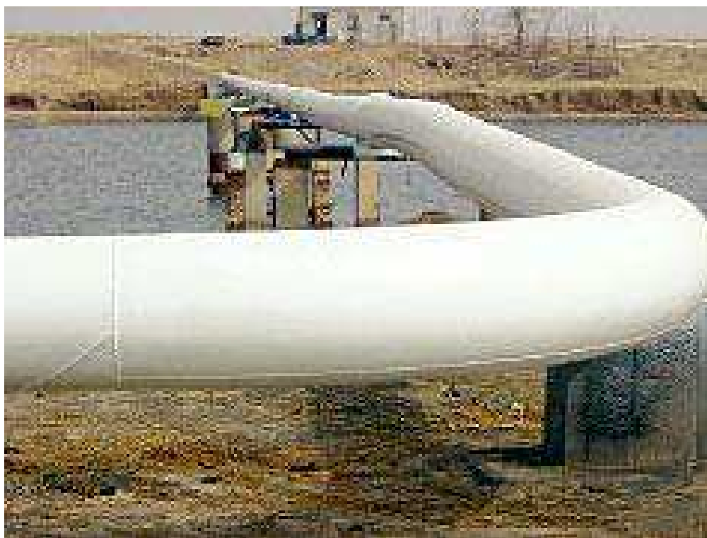
Photo 4 – Example of elevated LPG Pipelines crossing waterway
