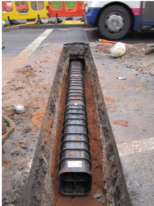
Photograph 46: Example of a Pipeline Protection Conduit
