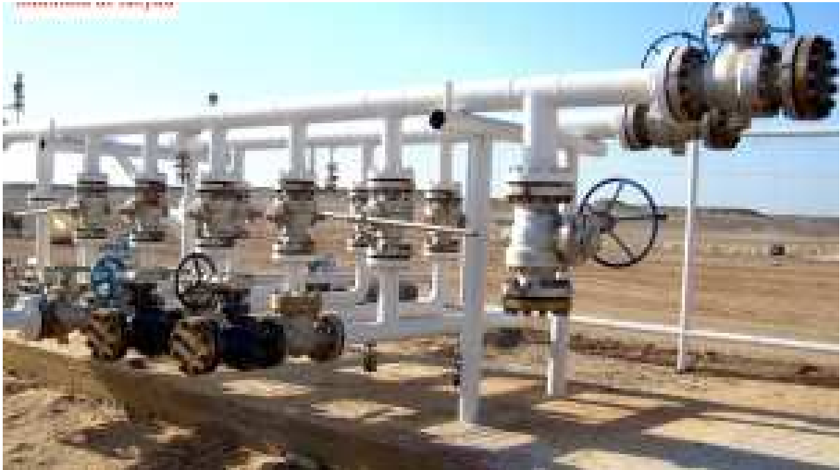
Photo #21: Example of a manifold system
