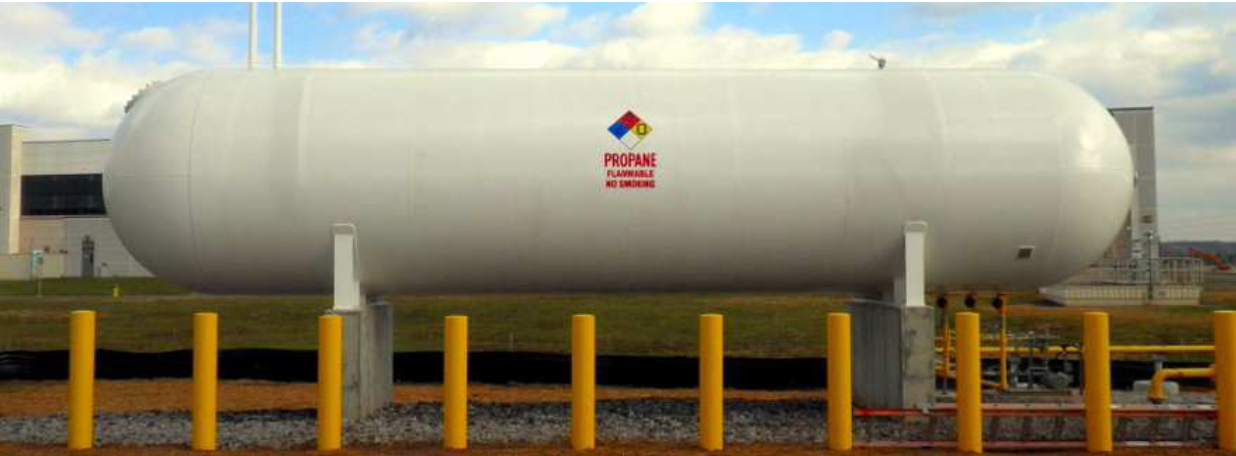
Photograph 20C – Protection Barrier/Pillars around LPG Tanks
