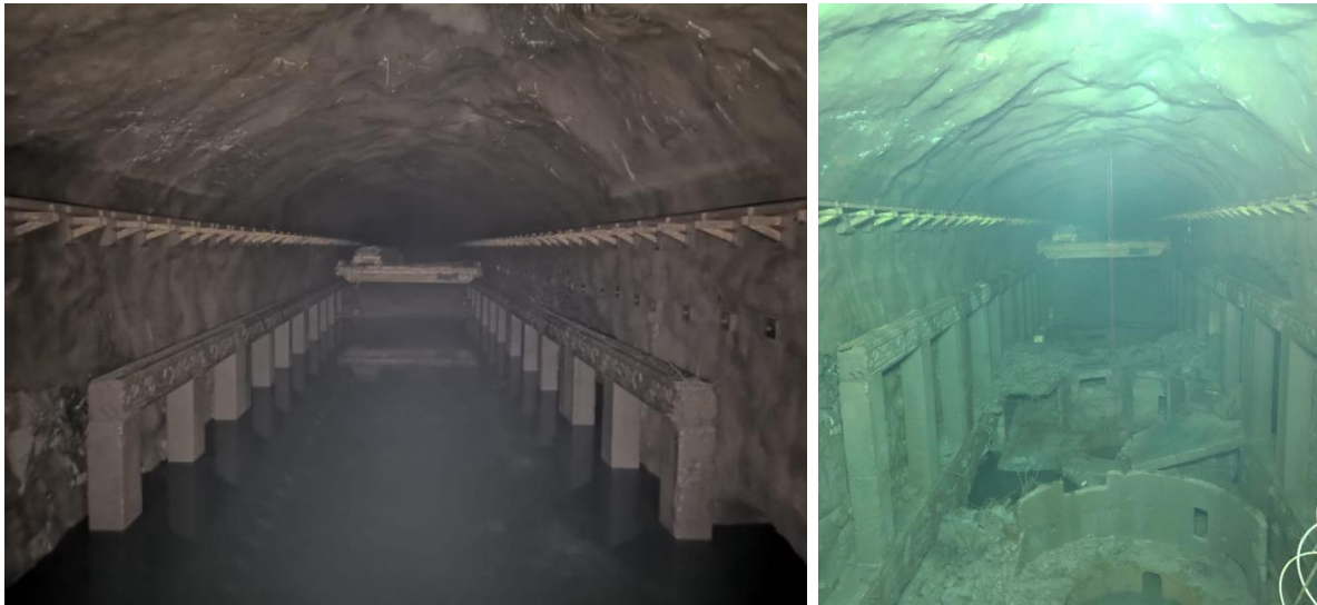
Figure No.6: The cavern of the Power House; in February 2019 (left) and March 2019. The fundamental geometry is conserved.
