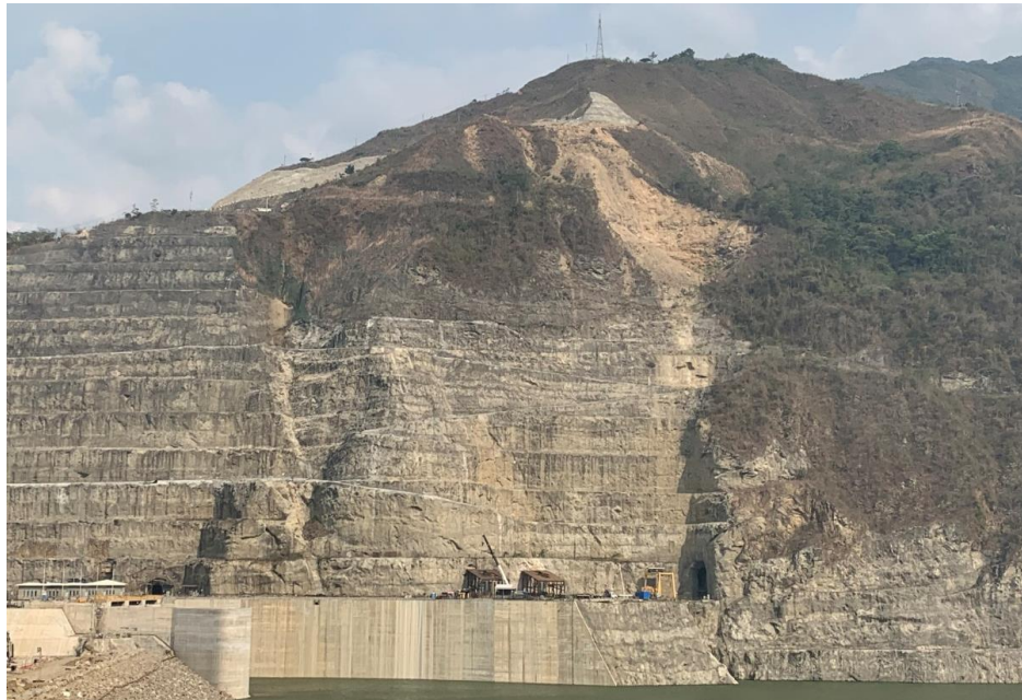
Figure No.12: The slope over the intake structures and the treatment works initiated uphill.
