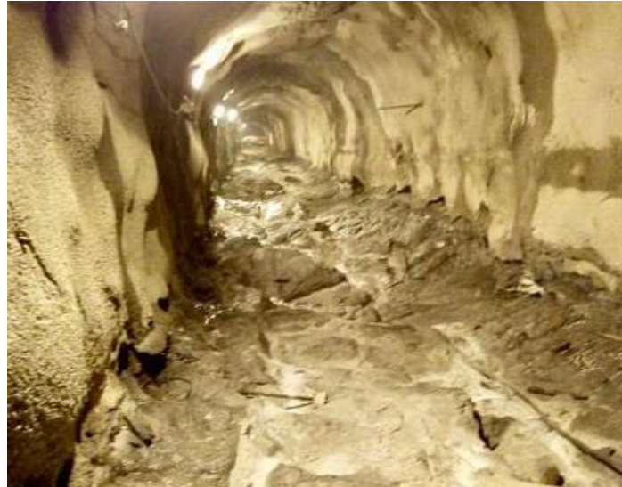
Figure No.4: An eroded and destroyed tunnel invert
