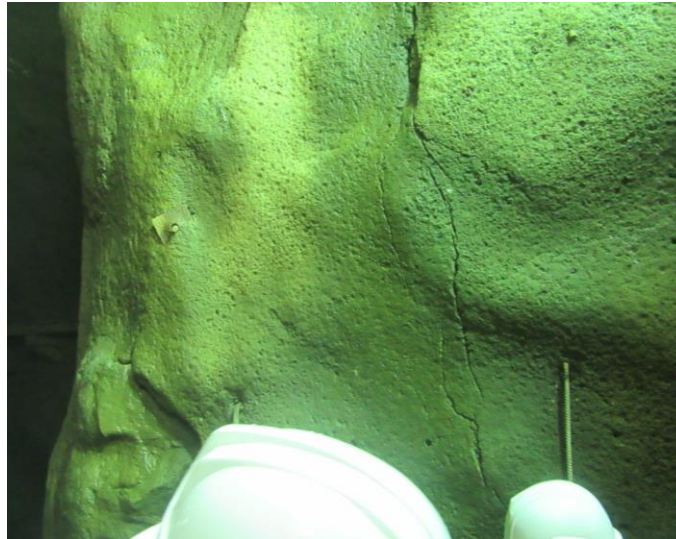
Figure No.3: Fissures in the corner of the access tunnel at the entrance to the power house cavern.
