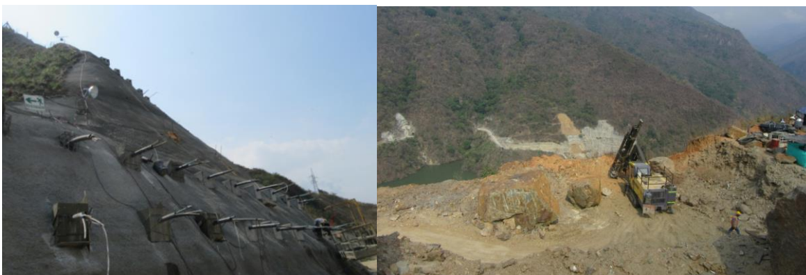
Figure No.13: The upper part of the “El Romerito” landslide under treatment with shotcrete and anchors. Benching down in the right photo.
