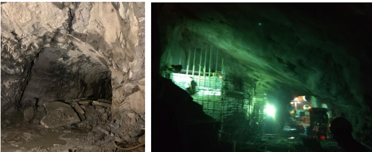
Figure No.2: Erosion and failure mechanisms - Wedges and slabs collapsed from tunnels' roof
