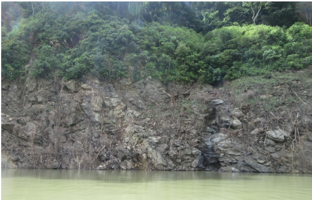
Figure No.6: Distressed gneissic mass, heavily fractured. Photo on the 2nd of August 2018
