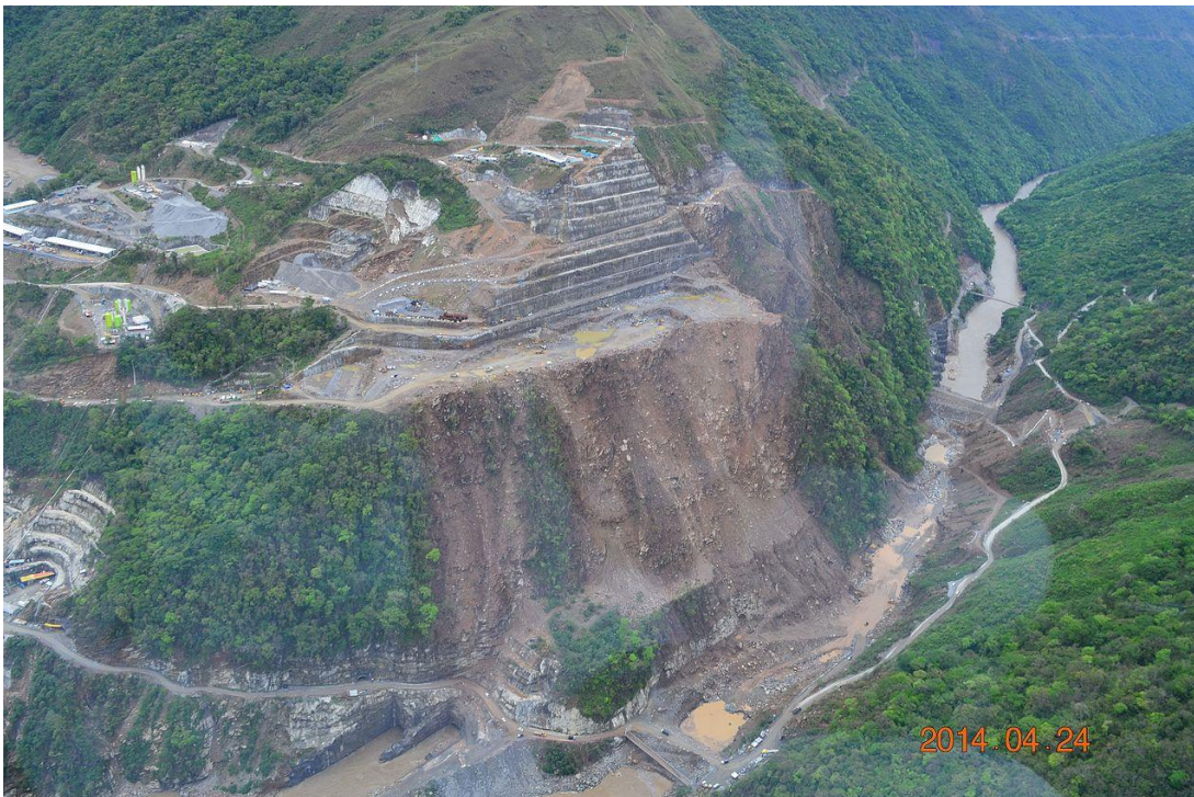
Figure No.8 The site of the project at the beginning of the construction, 2014. Skin slide on steep slope, behind the spillway cuts. In this area instability events occurred in spring 2018. Photo from Google.
