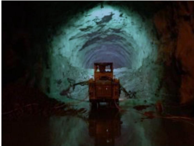
Figure No.3: Top heading and bench during construction of GAD. Small over breaks present (photo from the report of the Board of Advisors #12, February 2017)
