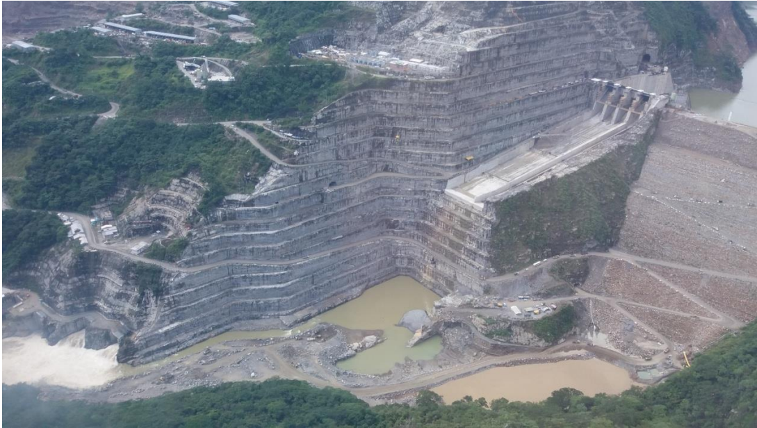
Figure No.9: Sound and good rock mass under the distressed zone on slope. Cuts for the spillway. Photo on the 3rd of August from the helicopter.
