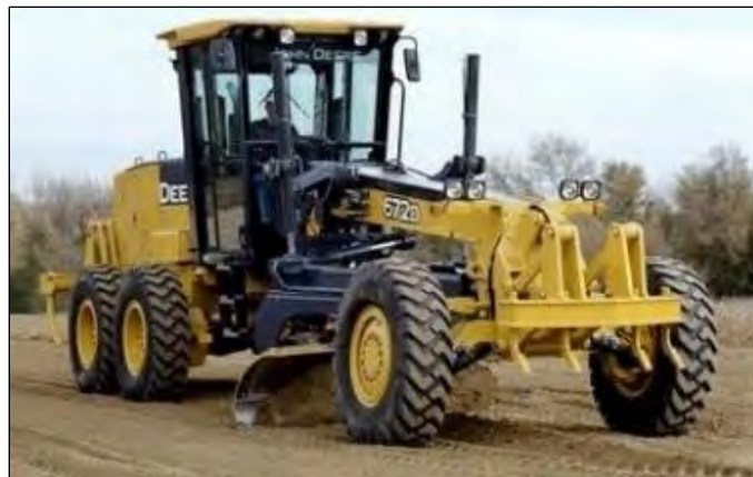
Photo Num. 3.6. Aeration of subgrade material when it has excess moisture Source: PIO SAS, September 2015.
