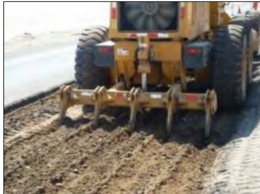
Photo Num. 3.4. Scarification of the surface of the subgrade Source: PIO SAS, September 2015.
